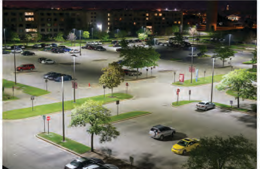
Optec LED Lighting provides Rosalind Franklin with a highly-efficient exterior lighting system that works toward its long-term sustainability goals
